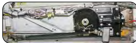
Figure 2-33. Power Distribution Unit
